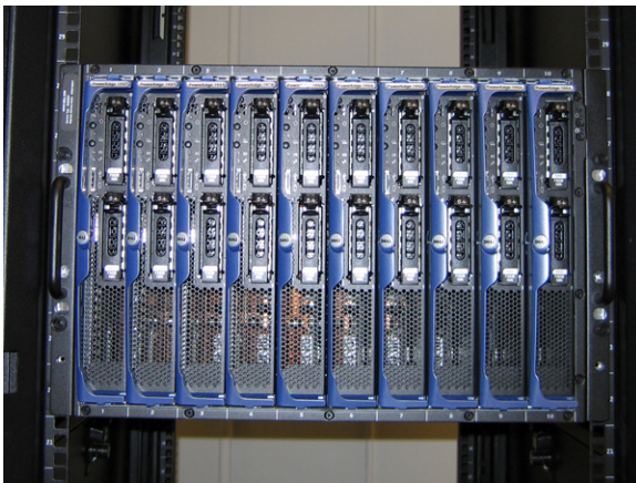
Figure 8A: The Dell blades installed in the chassis.
