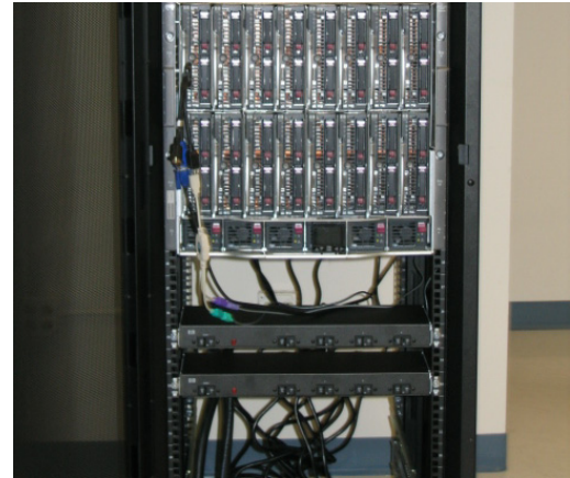
Figure 9B: The HP system with the PDUs installed.
