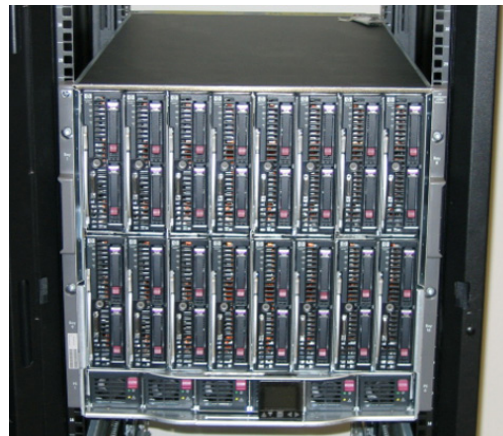
Figure 8B: The HP blades and power supplies installed in the chassis.
