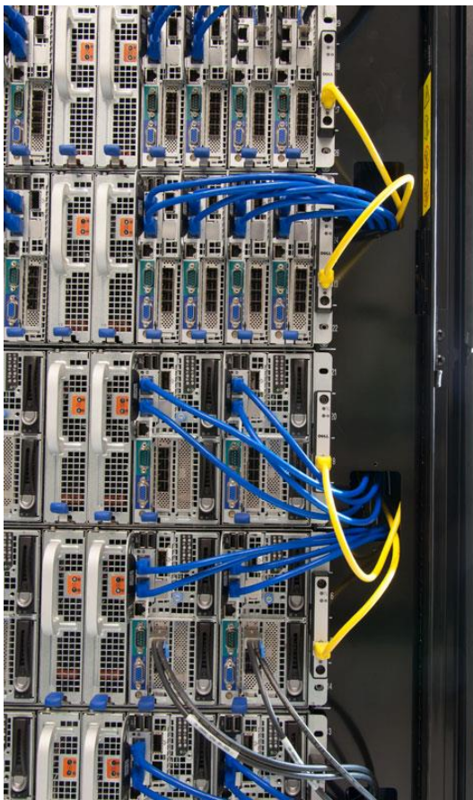
Figure 6: Management port Ethernet cable installation.
